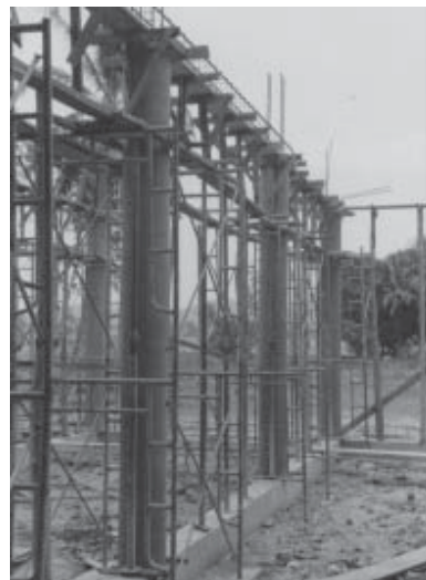
Figure 1. Example of reinforced concrete columns having asbestos cement pipe as permanent formwork
