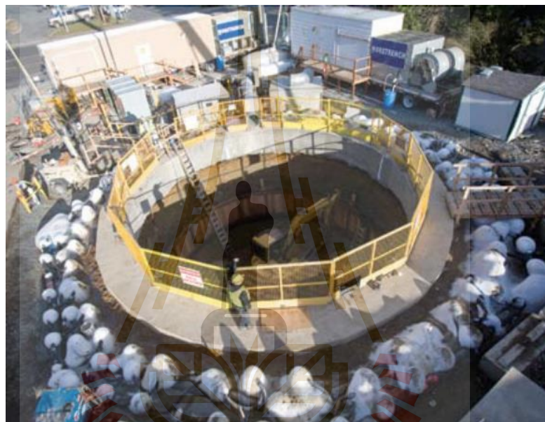
Figure 2.1 Construction of Brightwater Tunnel in King County, Washington, USA uses ground freezing method (More Trenching Machine excavator, www, 2014)
