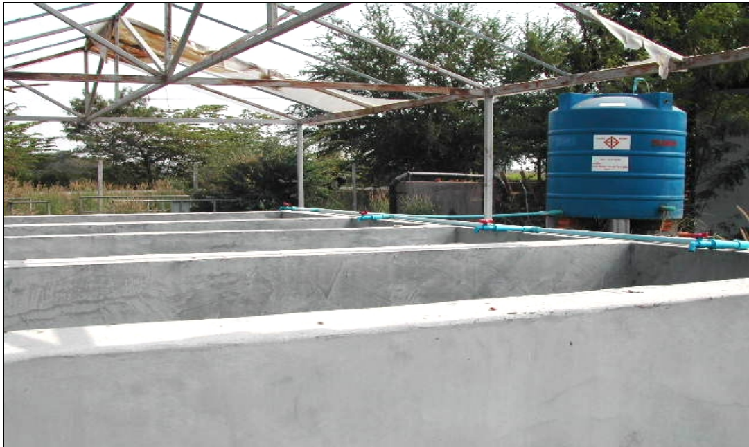
Figure 3.5 The reactors of waste stabilization ponds.
