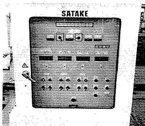
ฏ. Biomass Gas Control
