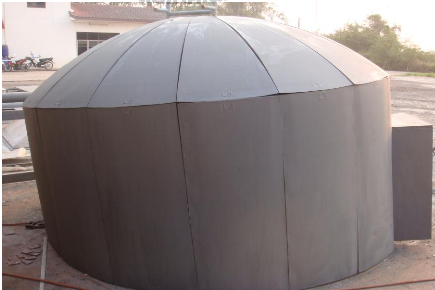
Attached figure 1 : the biogas digester and steel frame
