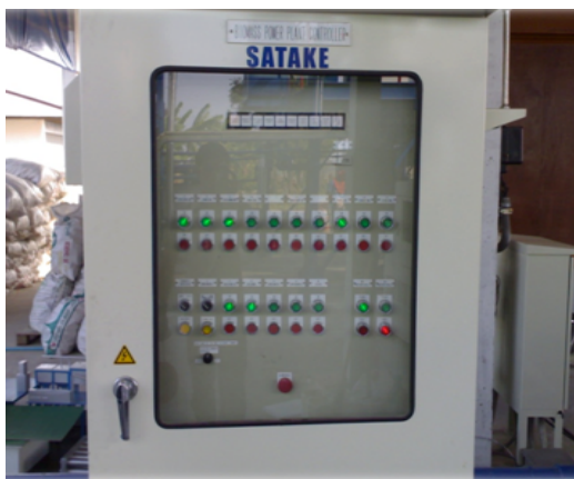
ณ. Biomass Power Plant Control
