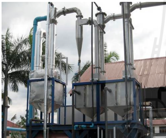
ค. Water Scrubber and Chiller Scrubber
